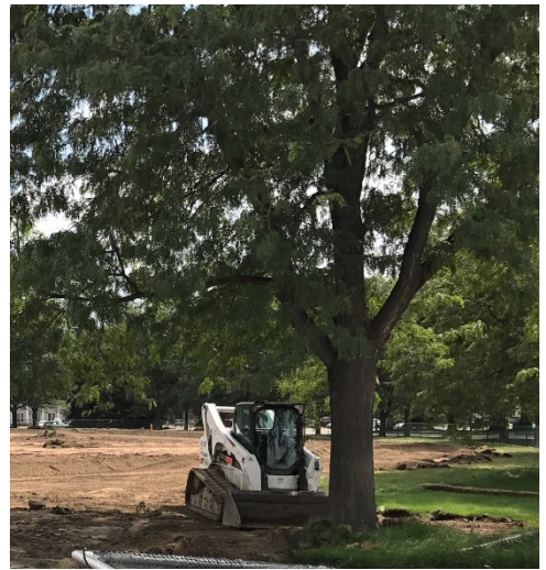
Heavy equipment traffic compacts soils
