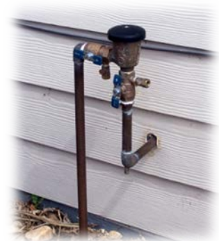
Figure 2. Required by local building codes, backflow prevention devices are typically located where the line comes outside from the house.
